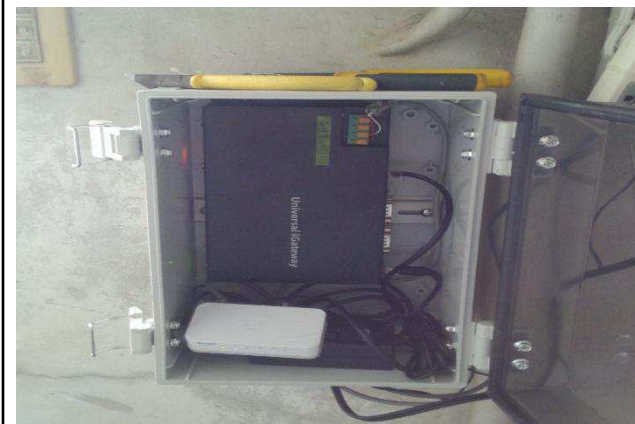
Smart Gateway communication wiring
