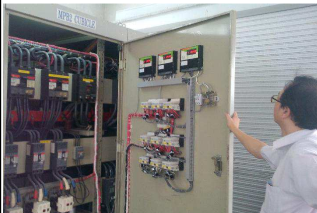
ST-12 Smart Meter power transmission test
