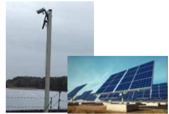
Solar Power Plant
